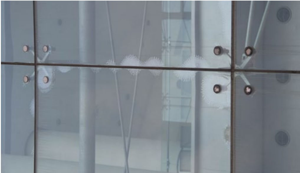
Typical defects caused by delamination.
