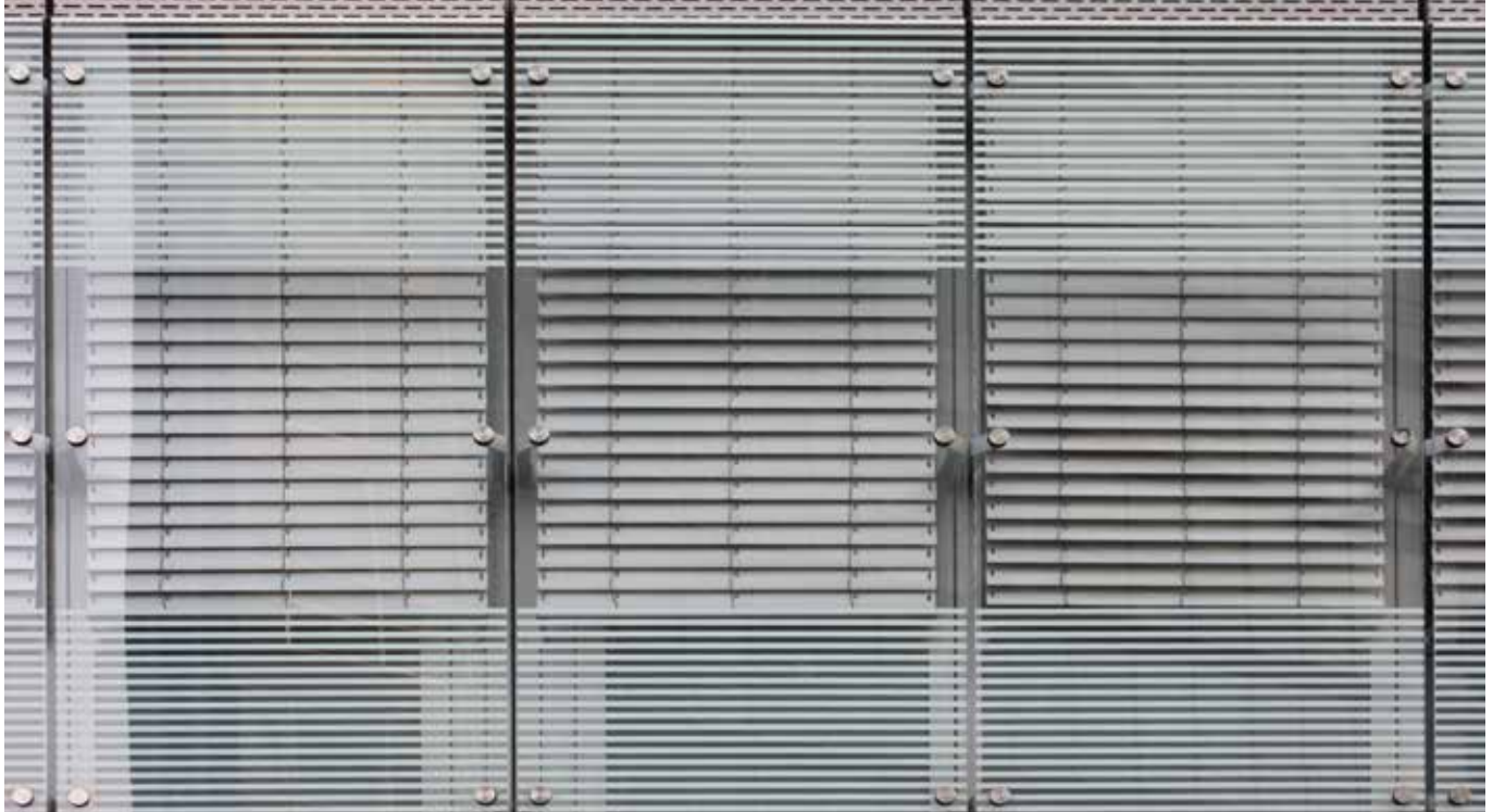
The individual point-fixed laminated glass panels of the Ares Tower's external façade each measure 1370 mm (54 ") x 3040 mm (120 ") and weigh 125 kg. The SentryGlas® ionoplast interlayer enhances load capacity without any additional weight or design compromises.
